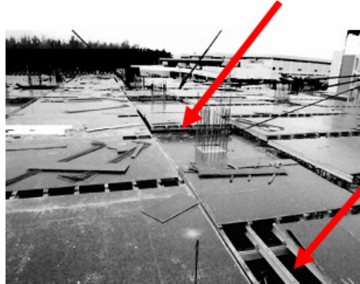
Figure 10: Lack of covering for open penetration (indicated by the arrows)
