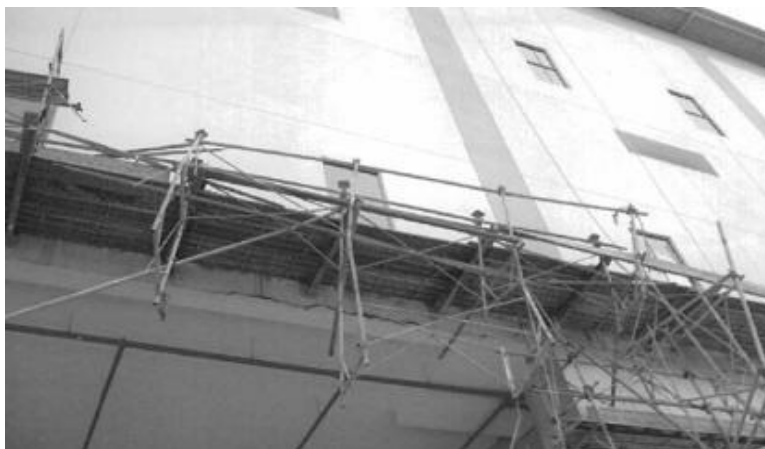
Figure 8: Poor working platform
